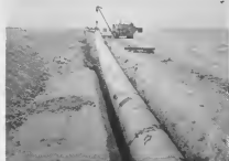
Side boom tractors lowering wrapped pipe into ditch along Tappin's right-of-way. The giant pipeline crosses some of the most varied terrain in the world.
